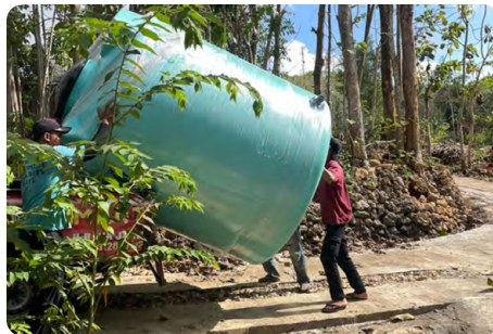
Installation of the GRF system: Transportation and installation carried out with the cooperation of villagers
