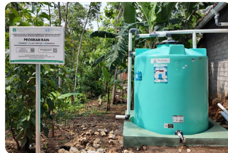
The installed GRF system
