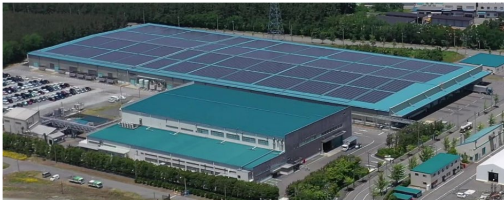
Photovoltaic power generating facility at Sakata Plant's production building
